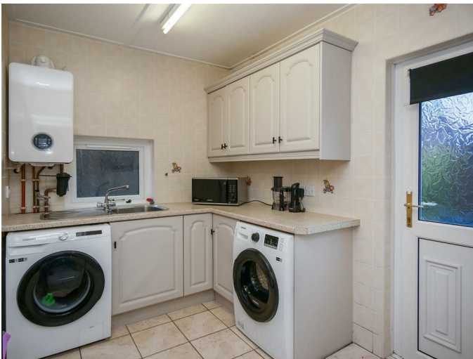
Range of high and low level units, plumbed for washing machine, single drainer sink unit with mixer taps, Part tiled walls. Tiled flooring. Housing Worcester gas boiler. Access to integral garage.
