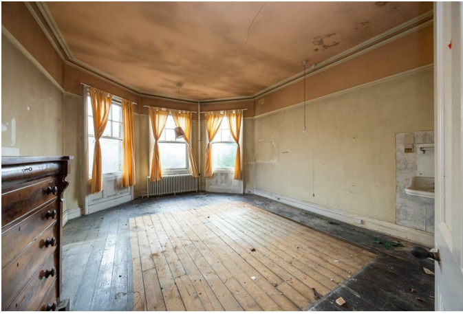
Bay window, pedestal wash hand basin.
