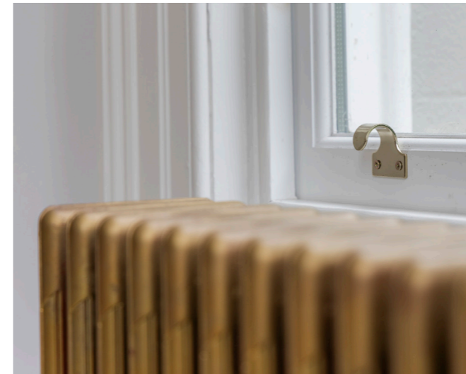
Cast iron radiators
