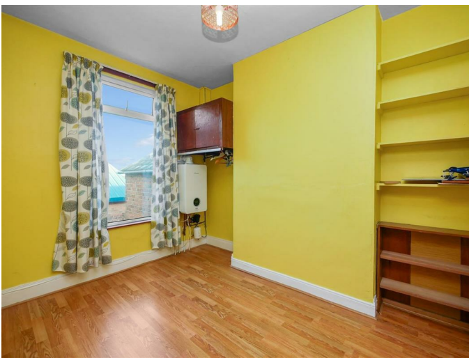
Laminate flooring. Gas boiler.
