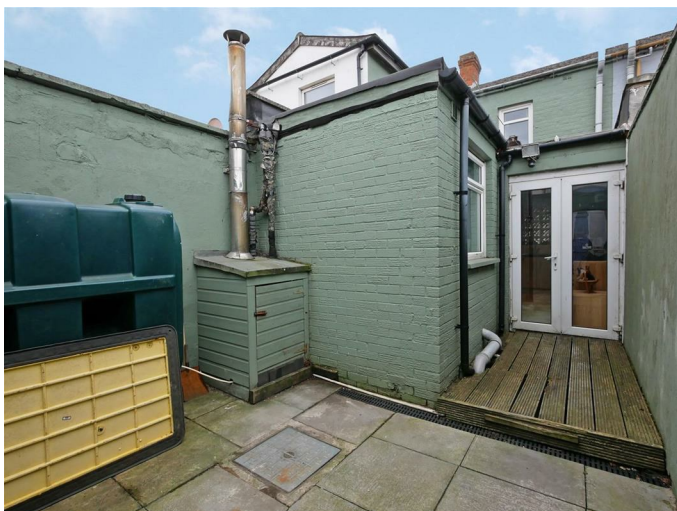
Enclosed rear yard housing oil tank and boiler.
