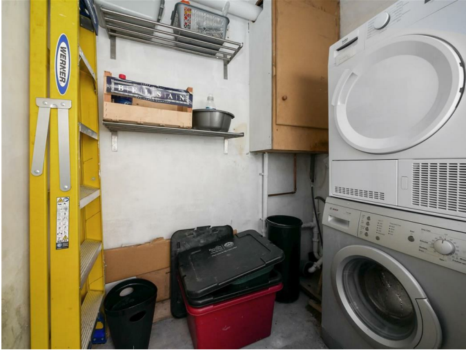
Utility area, plumbed for washing machine.
