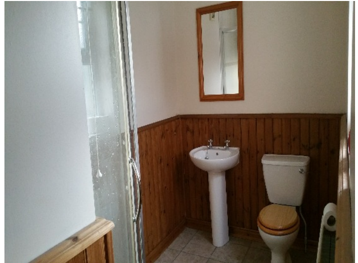
EN-SUITE - (7'11 x 5'11) to widest point, fully tiled corner shower unit with electric shower, low level w/c, wash hand basin, extractor fan, half panel wood walls, tiled floor
